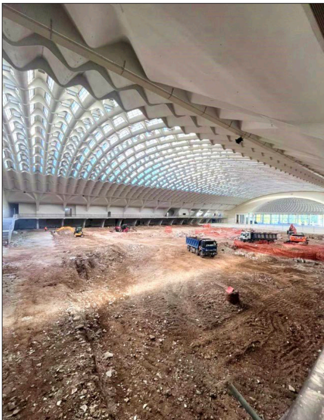
Fig. 1: P.L. Nervi: Pavillon B – Torino. Picture taken in the occasion of the visit organized in the Regenerate workshop carried out in Lecco (2023), in the framework of Recube project financed by EEC
